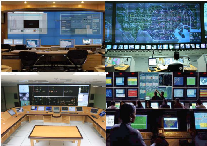
Fig.4 Examples of Monitoring Screen in Control Center
