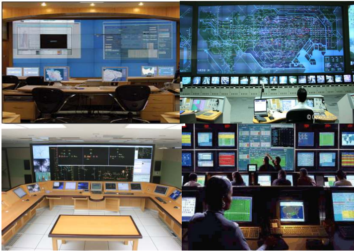
Fig.4 Examples of Monitoring Screen in Control Center
